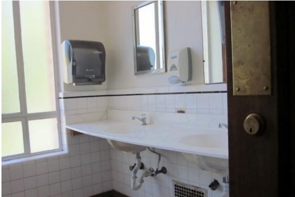
Men's restroom sinks
